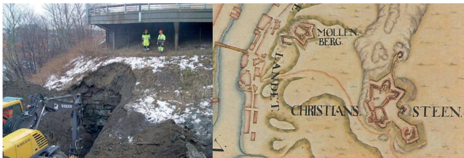
Figure 5.44. Left: Part of the revetment wall for the Møllenberg sconce/redoubt revealed in 2015. Right: The sconce/redoubt's location in relation to Kristiansten fortress in 1733. 801
