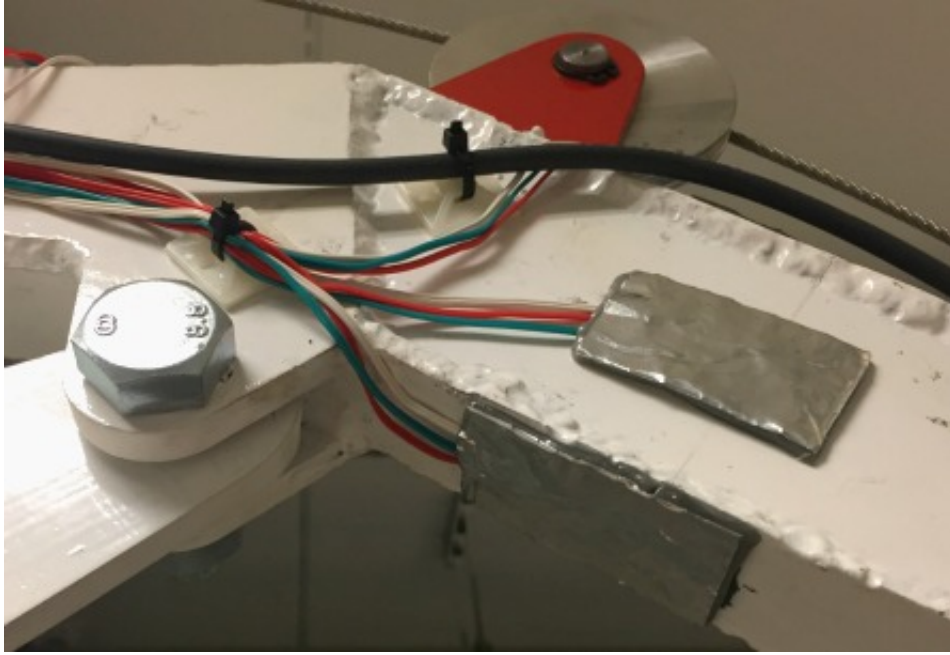
Figure 15: Strain rosettes on the crane
