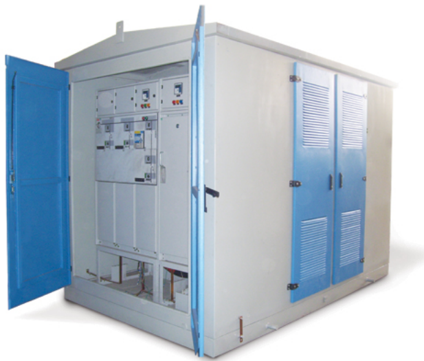
Figure 1: Compact substation with open front panel, showing the switchgear installed inside of it [1].
