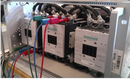
(a) Three sets of three phase contactors on grid converter and load sides.
