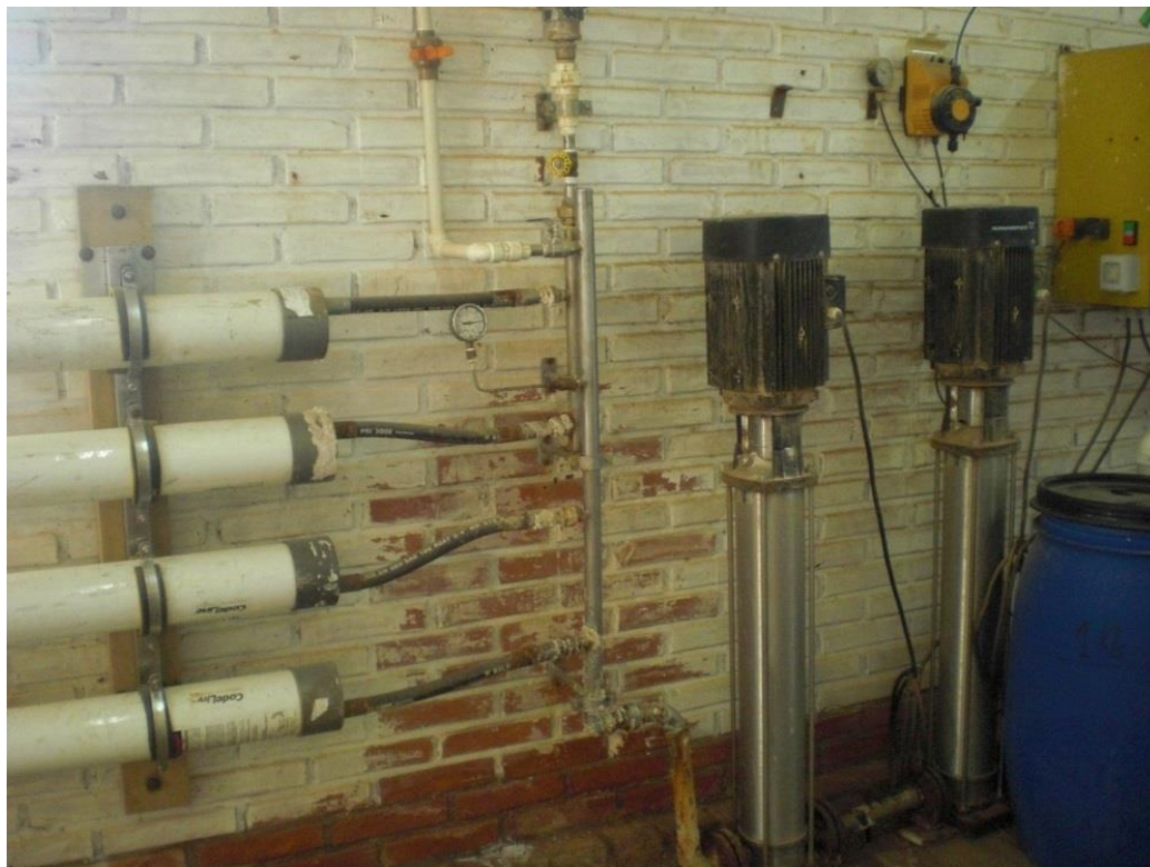
Figure 2.22 High pressure pumps and pressure vessels at Aguamin desalination plant
