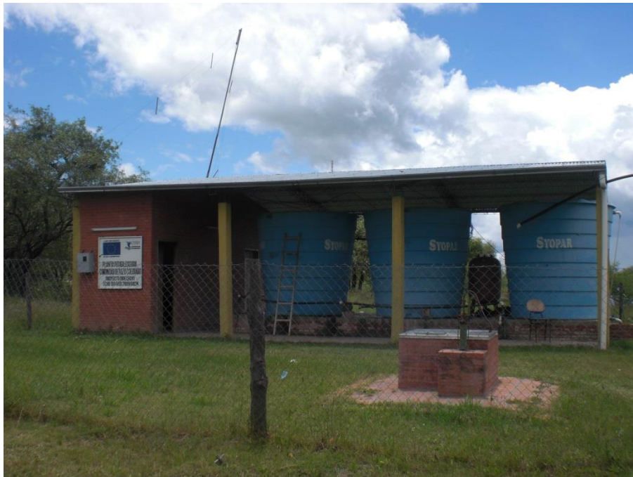
Figure 2.14 Three storage tanks of 10,000 liters each in Pozo Colorado
