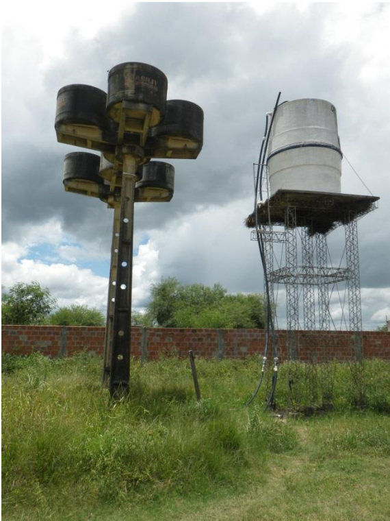
Figure 2.13 Elevated storage tanks in Pozo Colorado
