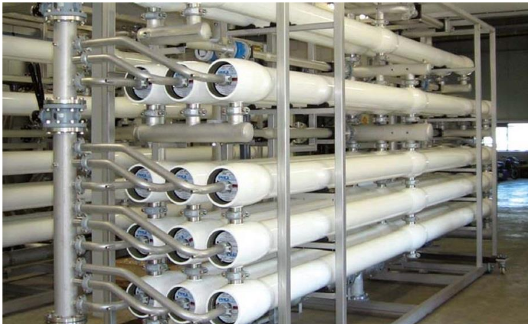
Figure 2.20 Pressure vessels containing RO membrane elements [26]
