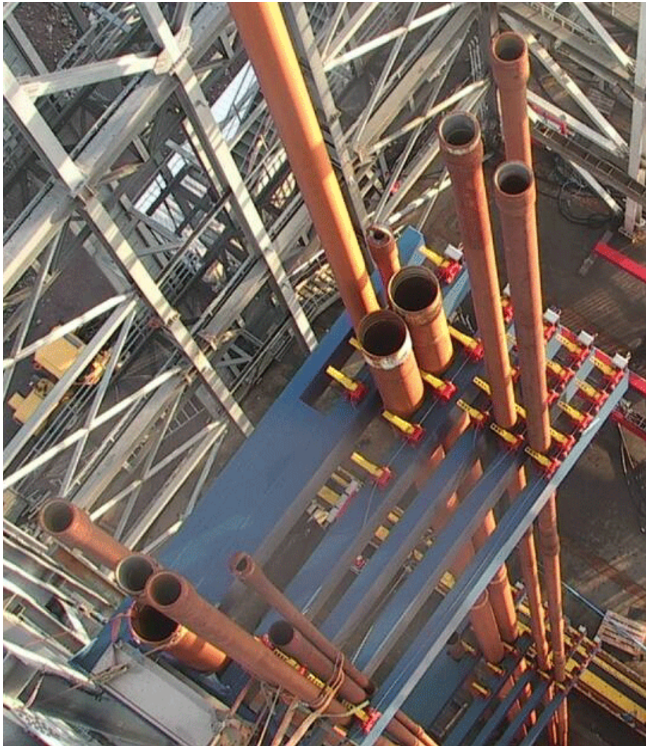
Figure 3.14: Fingerboard with tubulars. Source: Own work (MHWirth AS)
