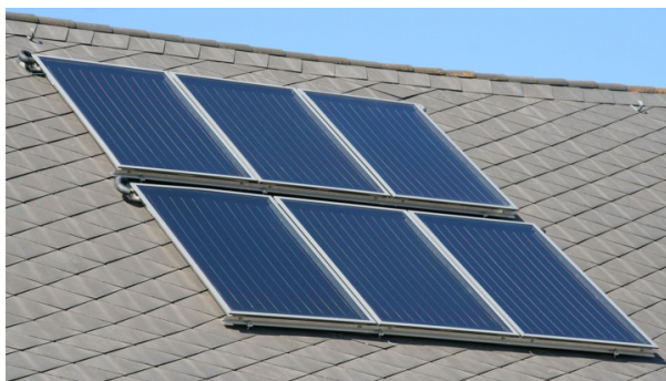
Figure 7-1: On-roof installation with flat plate collectors [30]
