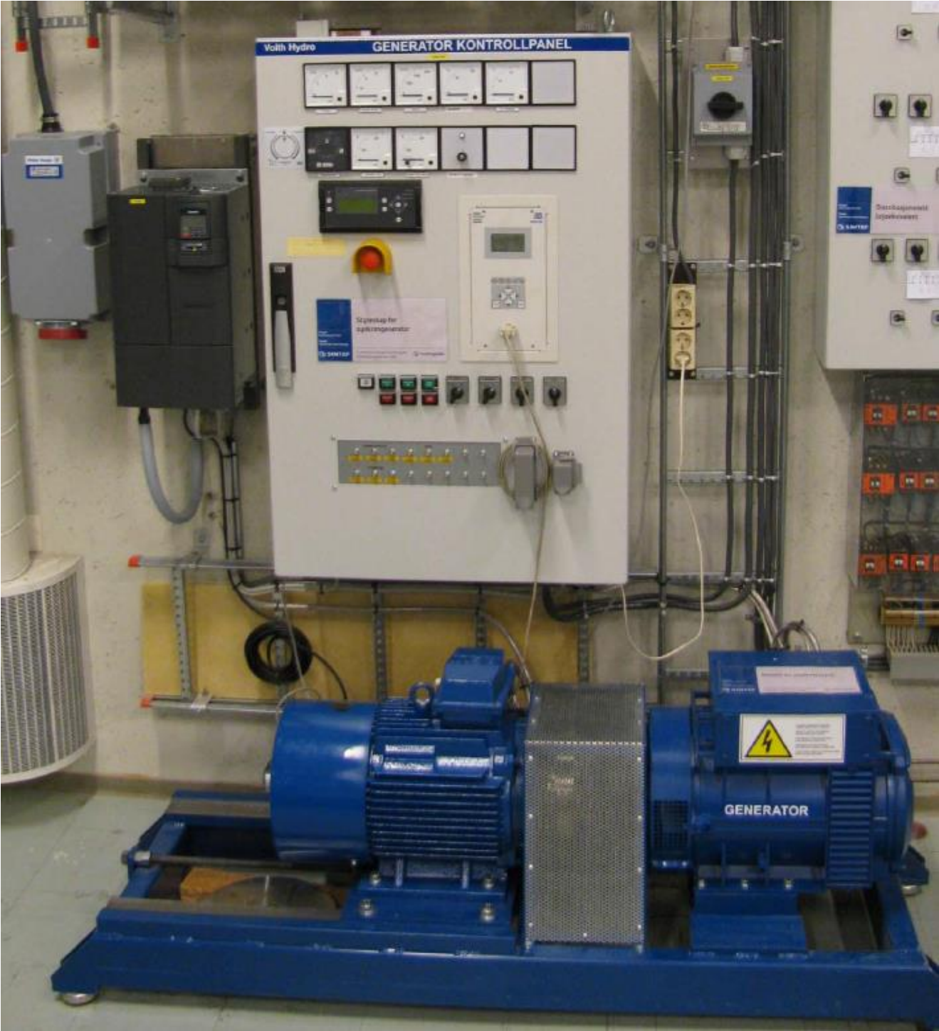
Photo showing the complete small hydro generation unit
