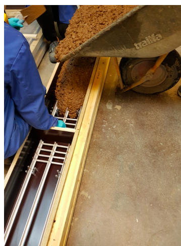
(b) Picture of the fresh concrete mix being poured into the formwork with corrosion protected reinforcement bars
