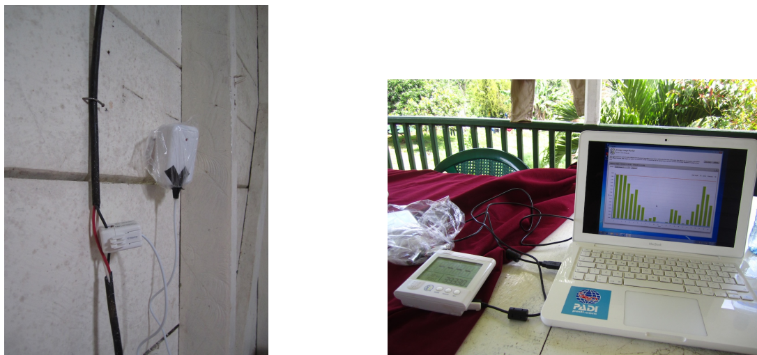
FIGURE 4.1: OWL+USB current meter Left: installed clumped meter with clamping sensor and transmitter Right: monitor plugged to a laptop and downloading data
