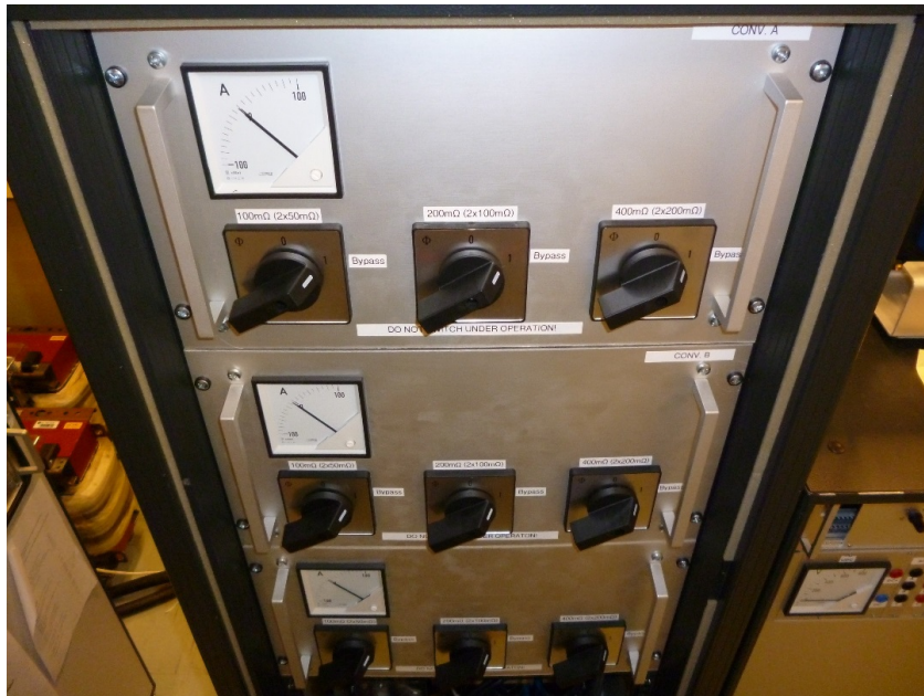
Figure A.3: DC resistors in the cabinet
