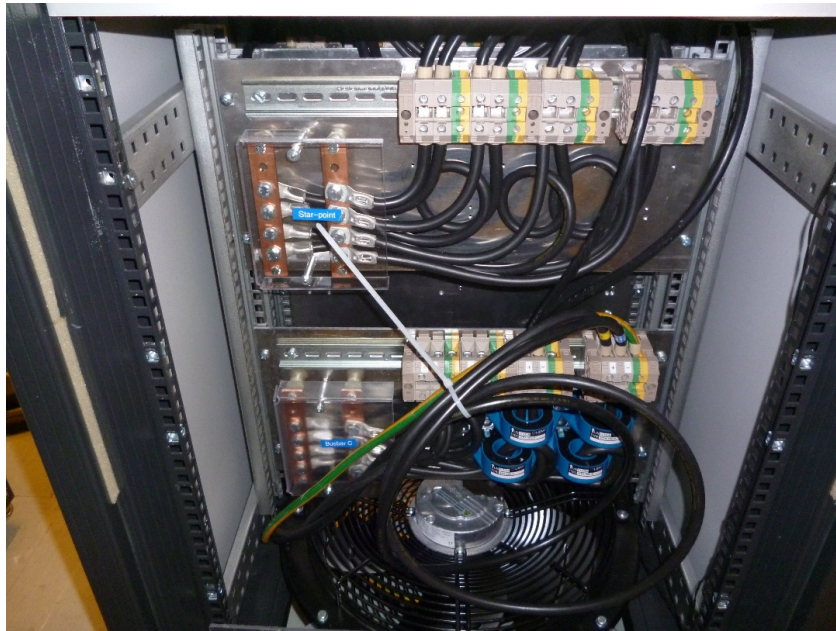
Figure A.4: Busbars and cooling fan in the cabinet
