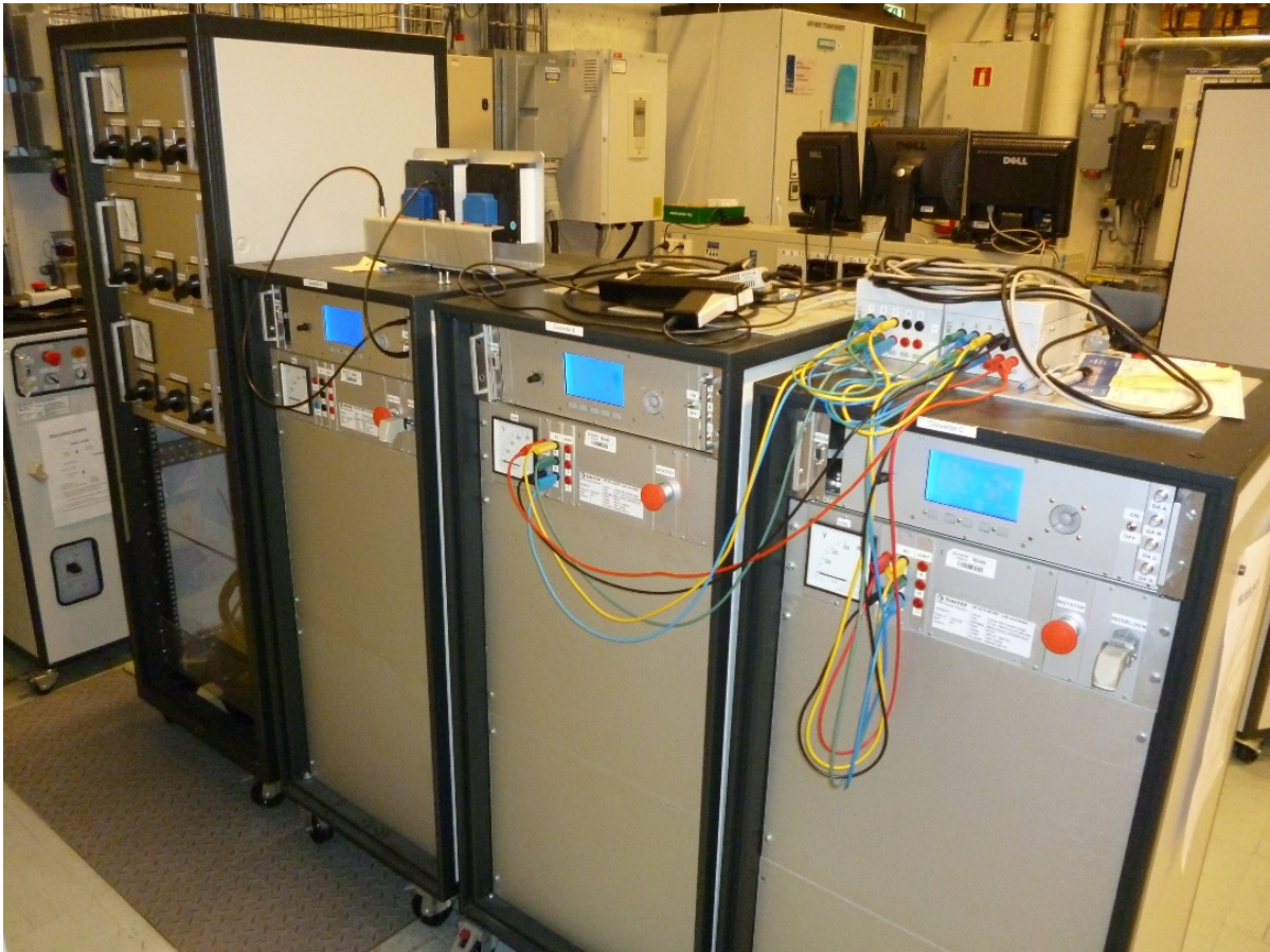
Figure A.1: DC resistor cabinet and voltage source converters
