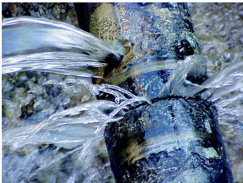
(Fig.2 Example of breakage)
