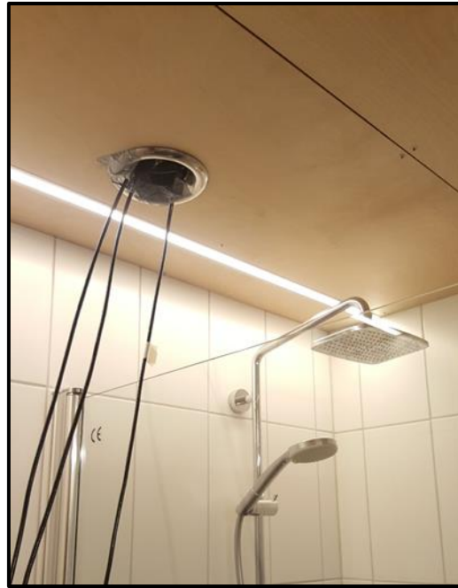
Figure 4.6: The calibration of the sensor type HMT333 was conducted towards the installed sensor HMT120 in the ventilation extract duct in the bathroom of Living Lab.
