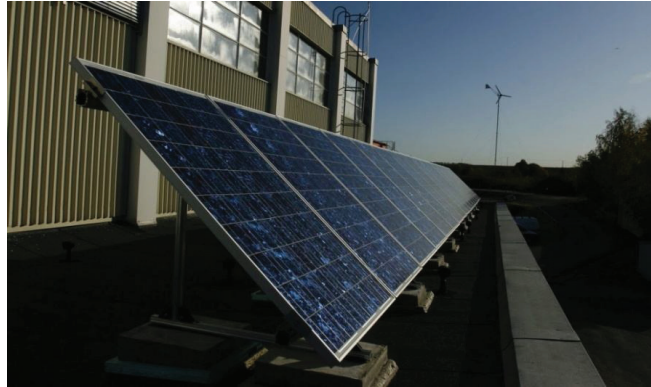
Figure 7- 2 PV array on rooftop
