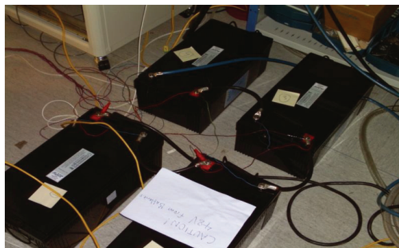
Figure 7- 5 Lead acid battery bank
