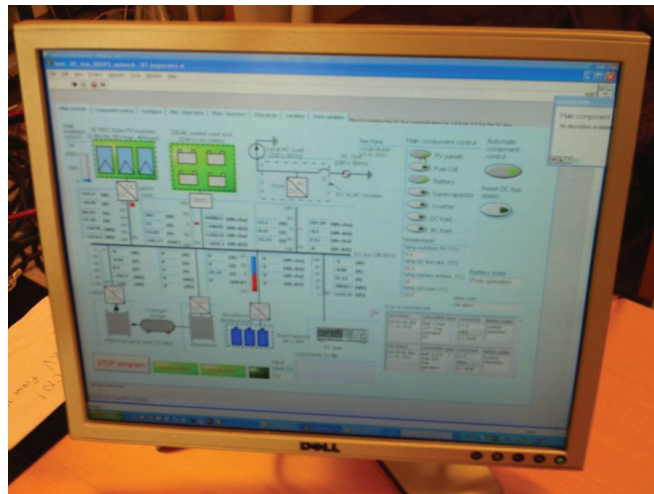
Figure 7- 8 GUI of test facility supervisory control
