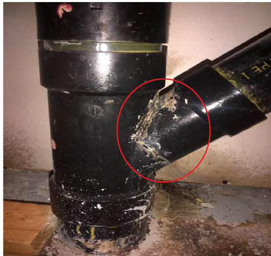
Figure 2.3: Cracked Pipe due to stress and fluid
