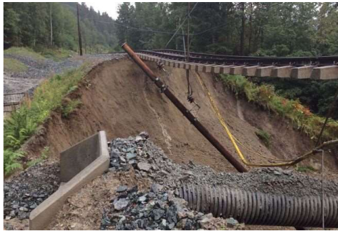
Figure C.1 – Lindelia debris avalanche, along with the Bergen railway. Photo by Jernbaneverket (Frank et al., 2015).
