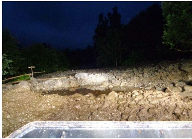
Figure C.70 - Picture of displaced material on road. Courtesy of Statens Vegvesen.
