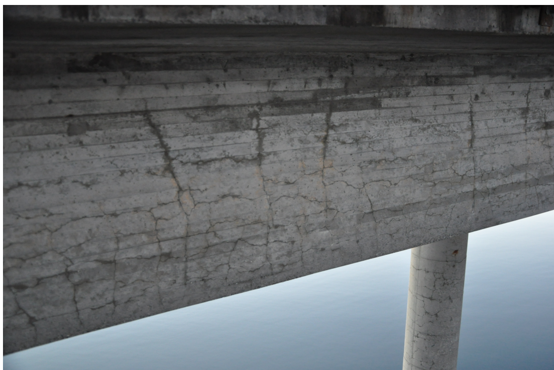
(a) Krakeleringsriss i bjelke
