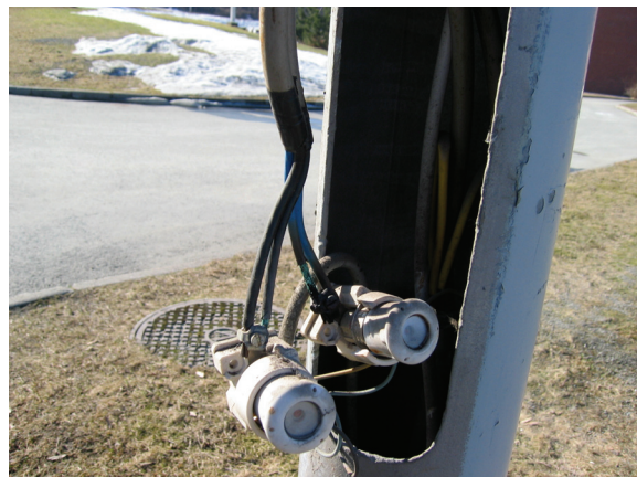
Figur 13-9: Patronsikringer (10 A) i mast
