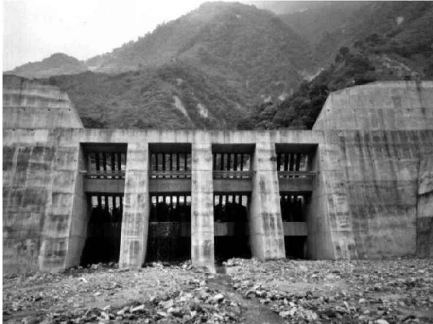
Figure 2-10: Sectional barrier with fins in Fong-Chiu, Nan-Tou County, Taiwan (Hübl et al., 2005)
