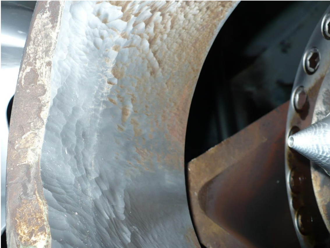
Figure 4.6 Nozzle wear due to sediments. (Source: El Canadá HPP)
