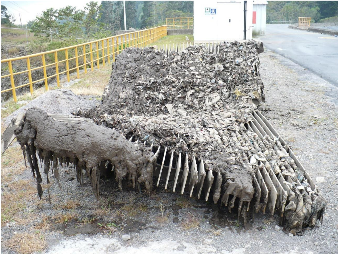
Figure 4.5 Damaged trash rack due to sediment clogging. (Source: El Canadá HPP)
