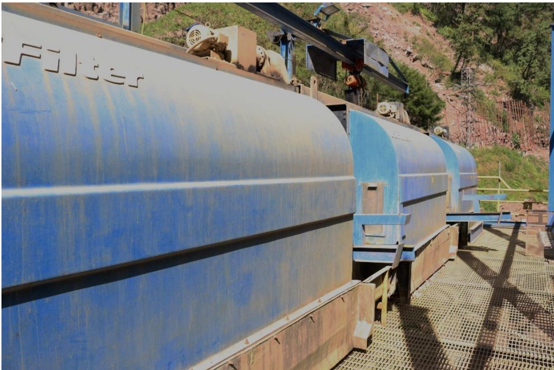
Figure 5.2 Garbage filters installed after the desander in El Canadá HPP's intake.
