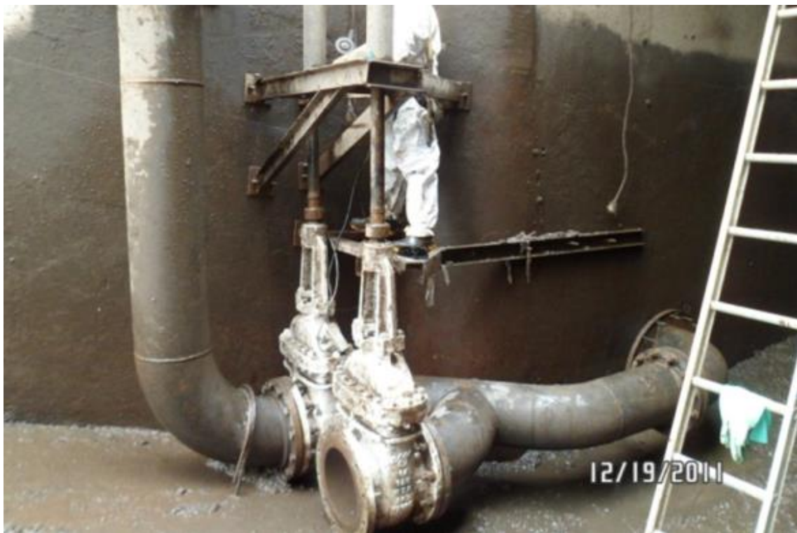
Figure 5.10 Bypass installation in the flushing pipe for connection of hydrosuction dredge (Jimenez & Figueroa, 2015).
