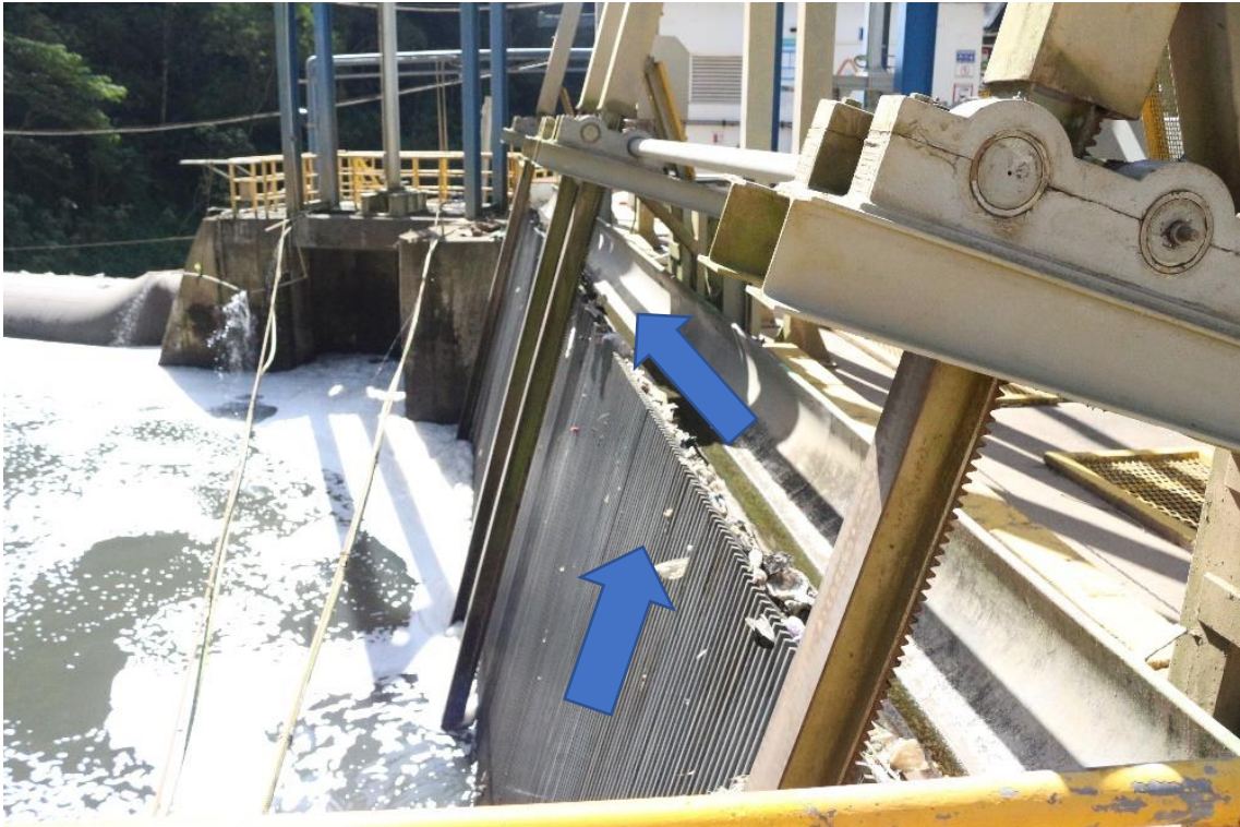
Figure 5.3 Trash rack with automatic collecting system in El Canadá HPP. The arrows show the path of the collection system.
