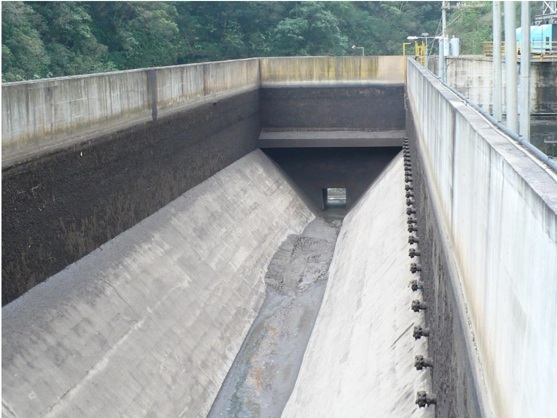
Figure 4.3 Flushing of sediments in the sand trap. (Source: El Canadá HPP)
