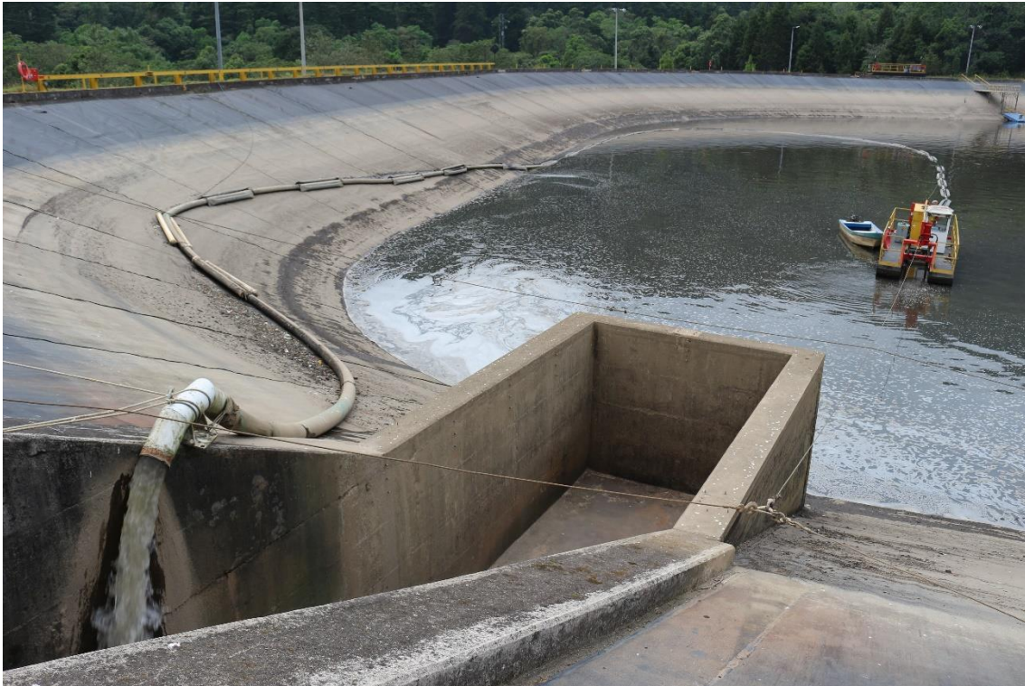
Figure 5.7 Diesel dredge arrangement and discharge.
