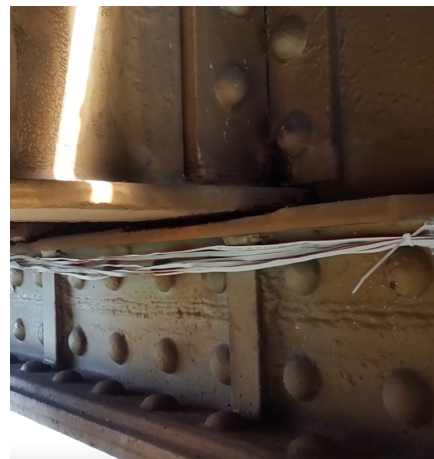
(b) Damaged structural component
