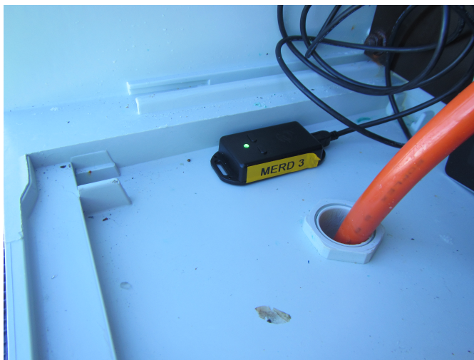
Figure A.13: Alignment of accelerometer inside power cabinet. All loggers are directed equally inside cabinets. Photo: Gunnar Senneset
