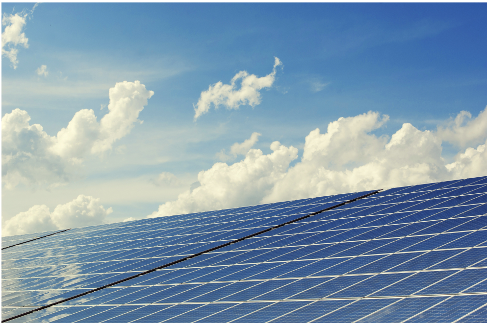
Figure 1.1: Example of Photovoltaic (PV) panels.
