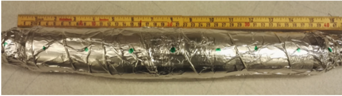
Figure 25: Picture of joint 3, readily prepared for acoustic PD localisation.
