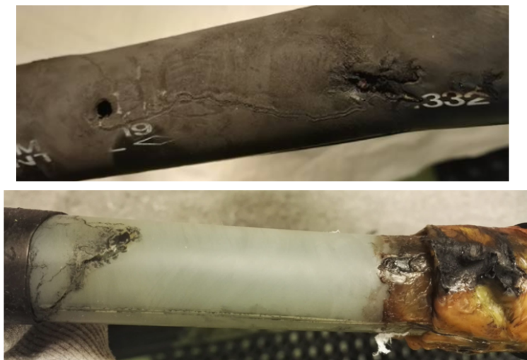
Figure 52: Above: signs of punctuation and tracking on the stress control tube. Below: signs of punctuation and tracking by semiconductor cut-off and on joint body.
