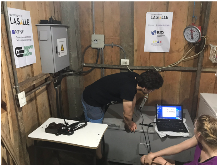
Figure 6.2: Installation Process in the refrigeration center
