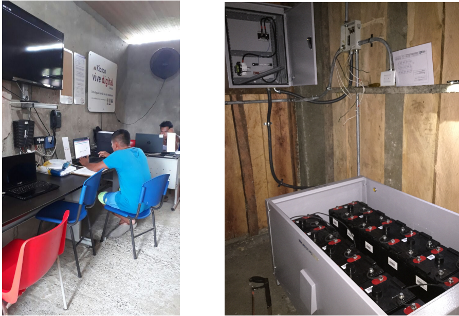
Figure 2.3: The digital kiosk in the school to the left and the installed equipment in the refrigerator center to the right.
