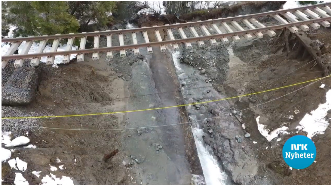
Figure 1.1 Embankment slide on the railway line Nordlandsbanen on the 22 nd of April after a blocked culvert lead to rising of the upstream water level (photo: Sivertsen, 2018).
