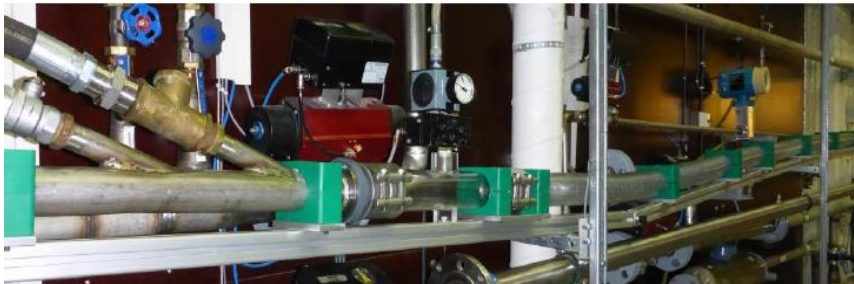
Figure2.26(a): S-riser nozzle was connected with a flexible pipe for a dip [3, p.35].
