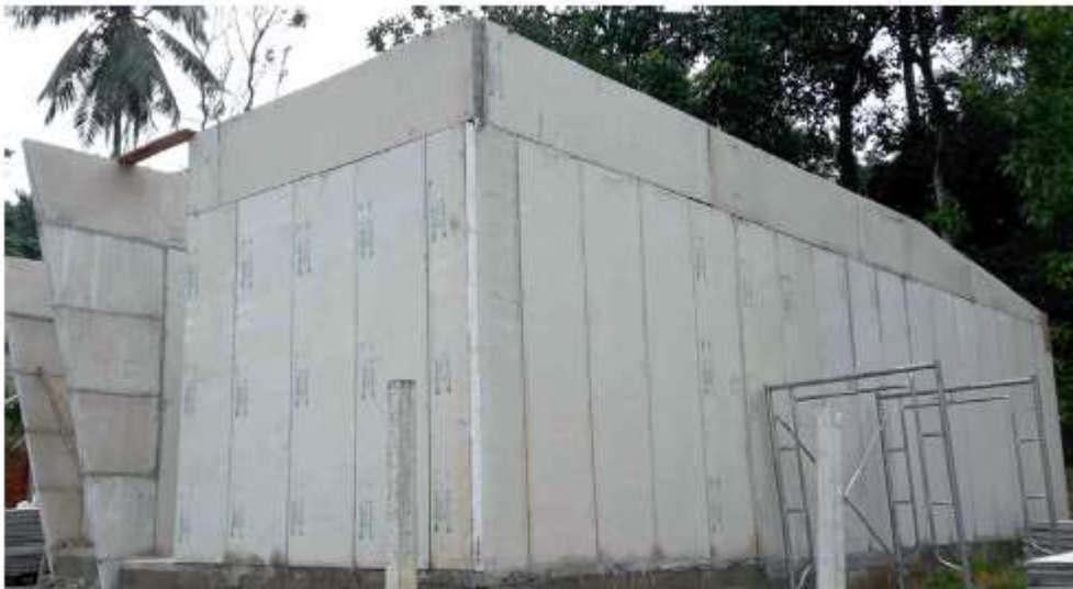
Fig. 8. Application of the EPS based lightweight concrete wall panels in a single storey house.
