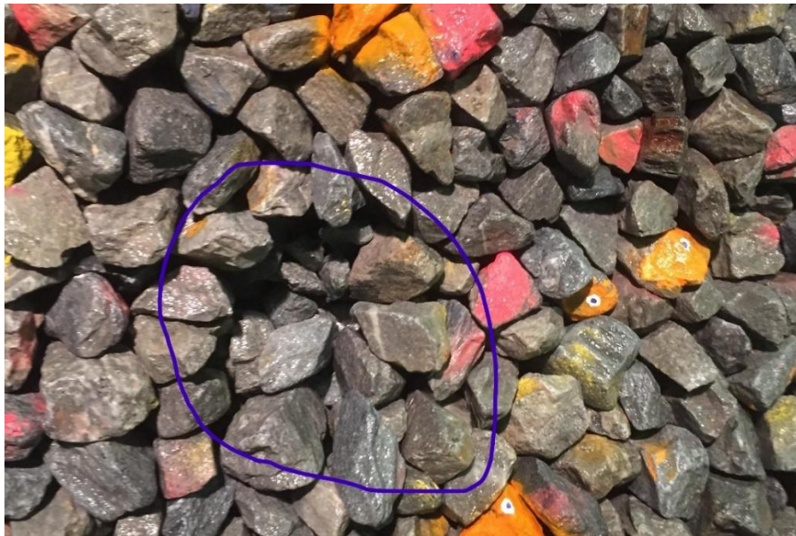
Figure 18 Removal of a single stone after one of the overtopping tests. Entire riprap structure worked perfectly even with that stone removed.
