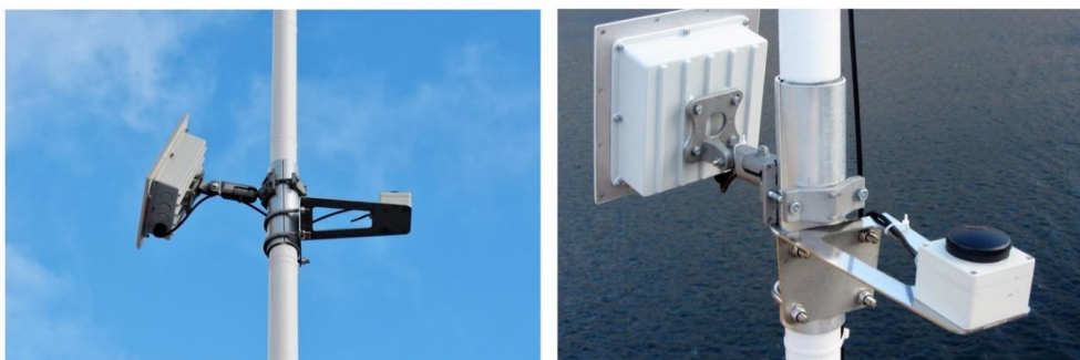
Fig. 12 Other instruments of the monitoring system: wi-fi antennas and GPS sensors are attached to hangers and connected to each logger unit. In both pictures, the antennas are on the left and the GPS sensors are on the right.
