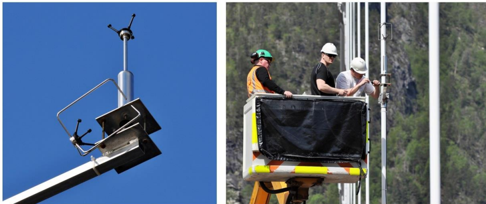
Fig. 13 Anemometer failure. The picture on the left shows the broken sensor. The head of the sensor is completely detached from its body; however, it is hanging on to the bottom plate by pure luck. The failure is believed to have happened due to fatigue caused by wild vortex-induced vibrations of the hanger. On the right: PhD candidates Øyvind Wiig Petersen and Tor Martin Lystad are working hard to replace the broken sensor.
