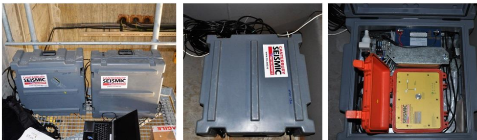
Fig. 11 Dataloggers at the Hardanger Bridge: on the left, two logger units at the Vallavik Tower are shown. The other loggers are placed inside the girder, close to sensors.
