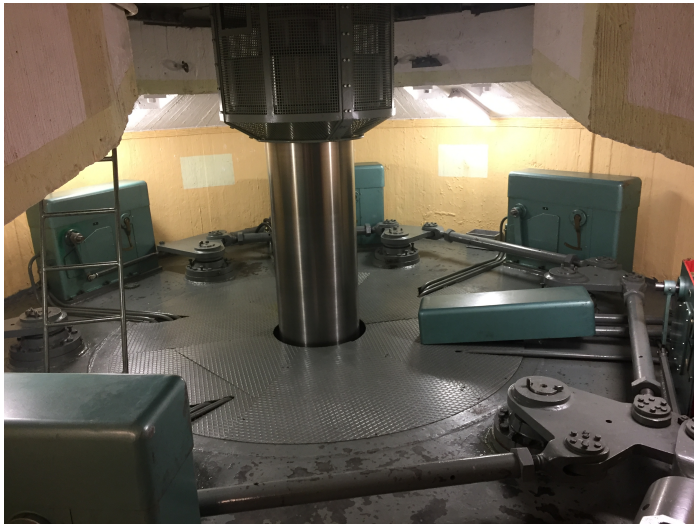
Figure 3.14: Turbine shaft and injectors
