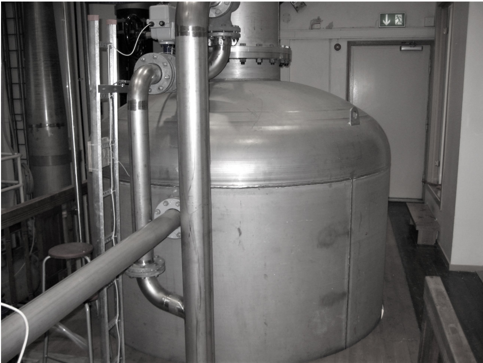
(b) Close-up of the top of the pressure tank, pipeline seen emerging at the middle of the picture.
