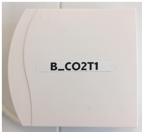
Figure A.6.: Sensor measuring the CO 2 level.
