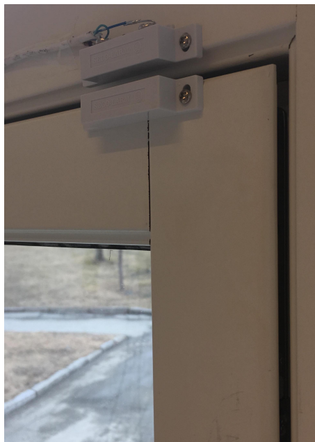
Figure 4.23.: Closeup of the window opening sensor. Photo: Stina Skeie.
