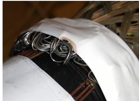
(b) The same arrangement as seen when the outermost layer of PVC tape with melted Armaflex was removed. The melted PVC with the strand short circuiting the arrangement can be seen in the middle of the picture.
