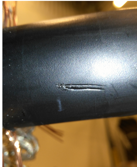
(b) Imprint from thermocouple on the outer sheath, where the force spring was placed.
