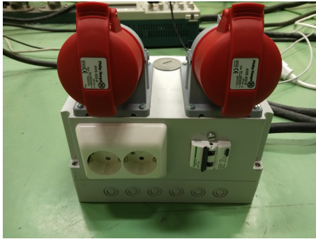
(a) On top: output for the DC sources. Bottom: Outlet to the control desk and variable voltage source (Schuko) with its circuit breaker to the right.
