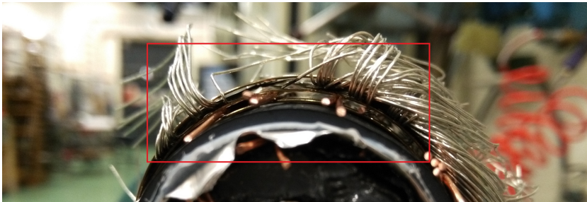
Figure 3.12: Picture showing the cross section of an incorrectly installed ground screen connection of type II. The cross section is taken from what would be the cable side of the joint in an installation. It can be seen that the copper wires and the joint ground screen is separated by a layer of the force spring (red box).
