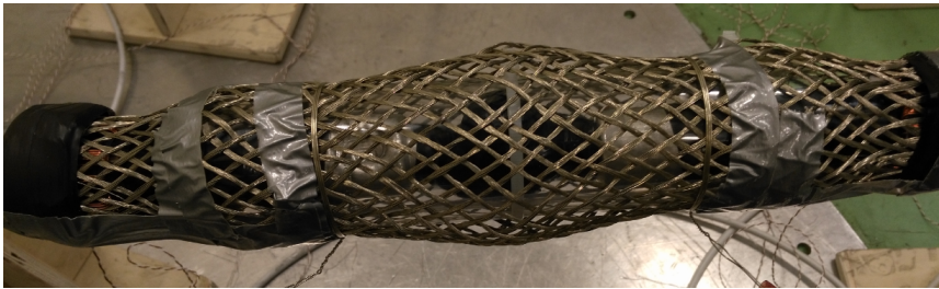
Figure 3.18: Figure showing the braided joint ground screen in place across the plastic tube covering the cable lug jointing. This picture shows the type I ground screen connection. The duct tape was applied to prevent the lead of the voltage measuring point to get metallic contact elsewhere on the screen.
