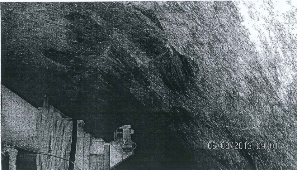
Figure 6: Rock slabbing/bursting around K16+545 under high stress condition.
