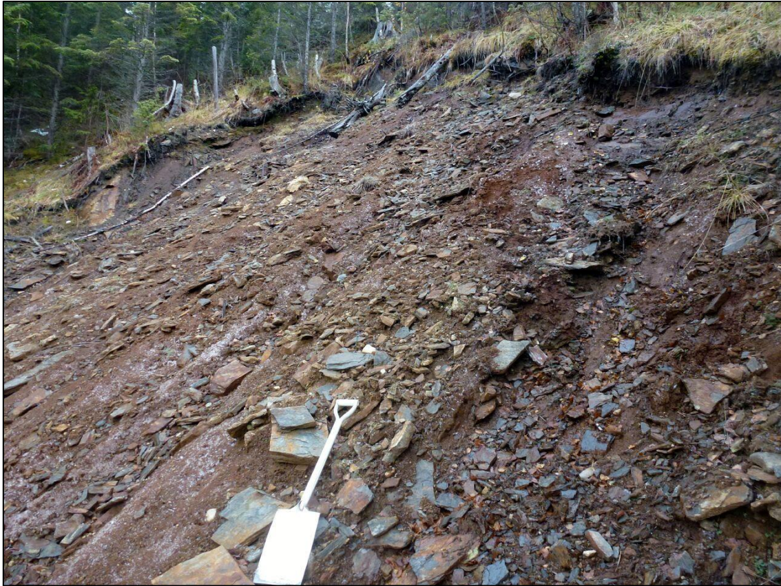
Figure 3.19: The back scarp of the channel in location 4.
