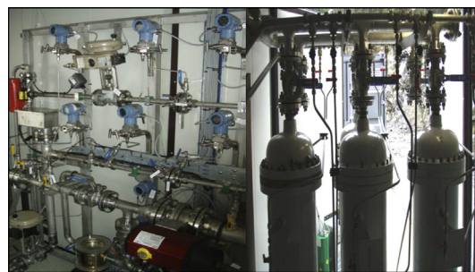
Fig. 4. Photographs showing the biogas upgrading membrane plant.
