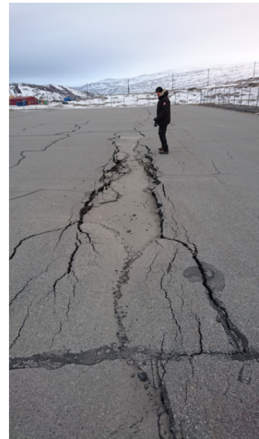
Figure 1.2: Thaw settlements and cracking at Kangerlussuaq airport in May 2017
