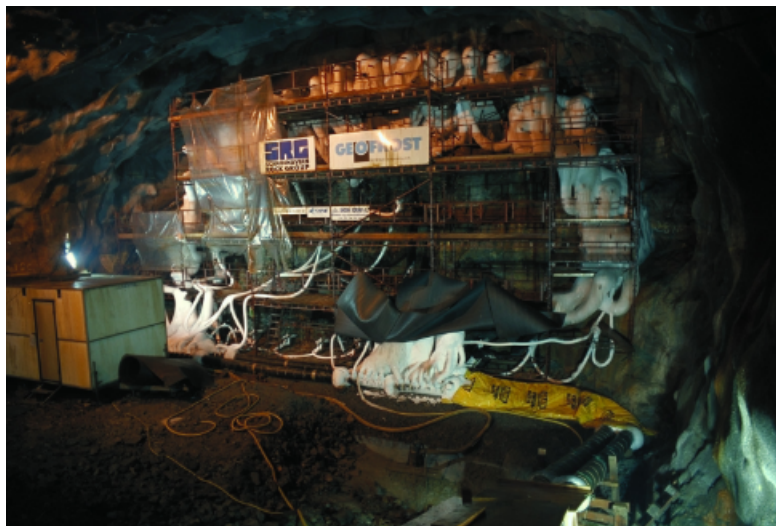
Figure 1.12: Freeze pipes installed at Oslofjord tunnel for crossing the weakness zone (GEOFROST, 2018)
