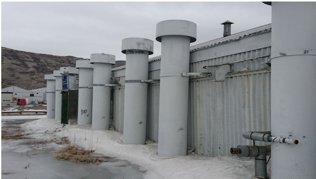
Figure 1.11: Thermosyphons installed in Kangerlussuaq to prevent permafrost from thawing beneath the buildings when the airport of the town was used as an American base during the Cold War. Photo taken in May 2017
