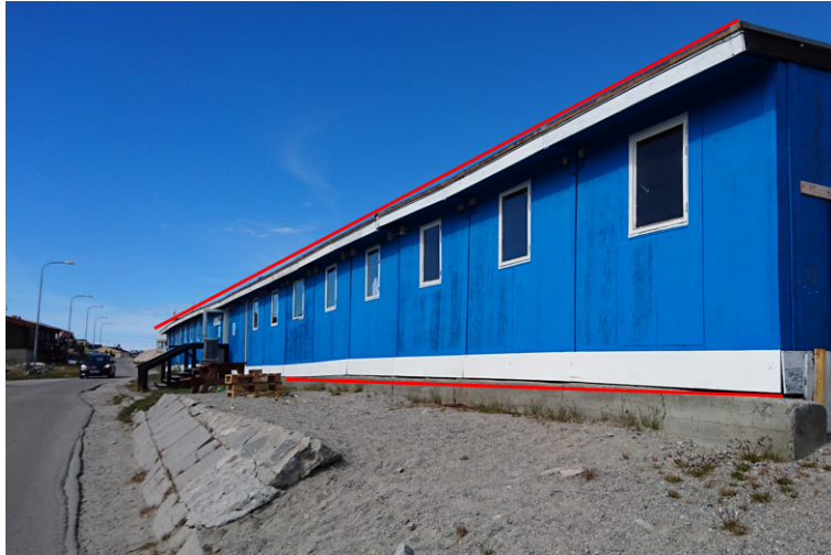
Figure 1.1: Building in Ilulissat (Greenland) visibly deformed due to thawing permafrost
