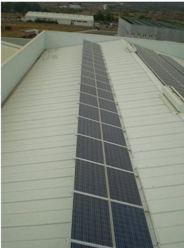
Figure 3 Example: Solar Energy Installation
