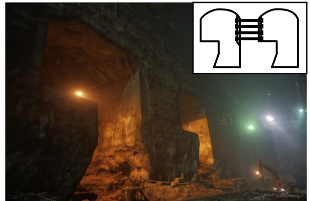
Fig. 23. Tieback bolting in a hydropower cavern. Some of the pillar-through cablebolts are shown in the picture (Photo by J. Mierzejewski).
