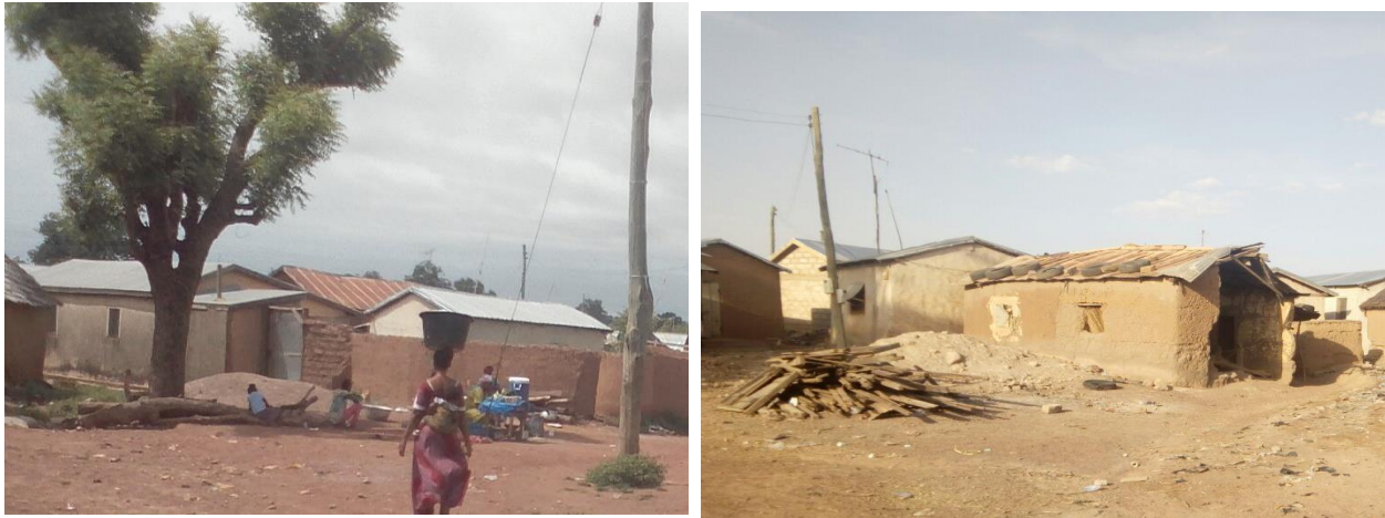
Figure 7.6. Photos illustrating poor housing structures in Fongni, unplanned area. (Source: Author work during the fieldwork).
