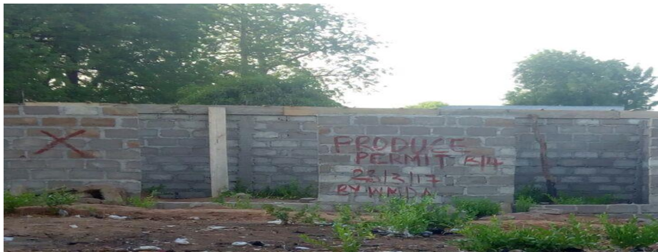
Figure 7.4. A photo showing non-building permit by a developer in Nayirifong, Walewale. (Source: Author. A picture taken during the fieldwork).
