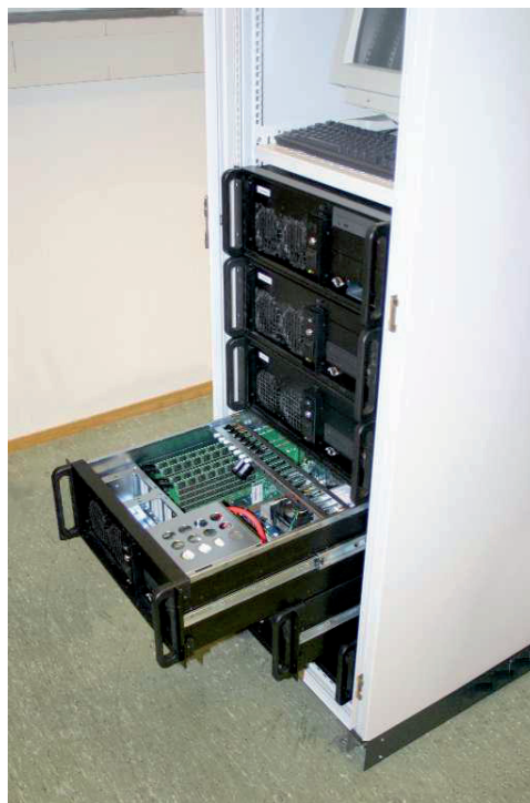
Figure 5.2: Rack of five nodes, containing 480 PMC chips operating in parallel.
