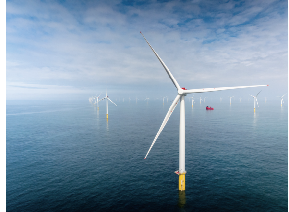
Fig. 5. Dudgeon offshore wind farm with 402 MW generation capacity located in the North Sea, England (photo: courtesy of Statoil).
