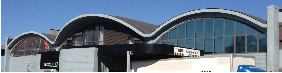
Figure 5: A1962 original building with different window types. The window area far left have original wooden frames, the middle area is probably a newer wooden Al clad frame with Al blinds, while the far right area consist of modern aluminium profile windows. It might also be that the middle and right areas are both Al profiles, but of different type, time or producer.
