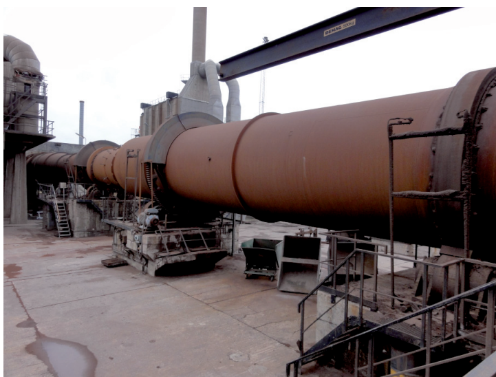
Figure 7-1: Used rotary kiln (Nr. 4) from Hinge plant in Denmark for production of calcined clay
