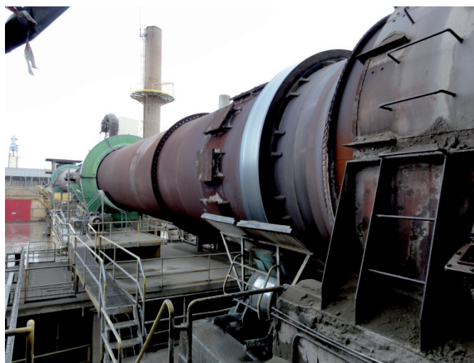
Figure 7-10: Kiln nr.2 at Avelar plant in Portugal
