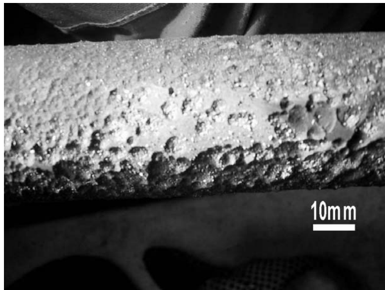
Figure 1.1 Example of pit formation on a drain line of a nickel-based alloy located in a steam superheater caused by metal dusting corrosion.
