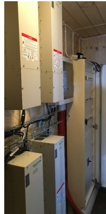
Figure 4.15 The Solar Charge Controllers in the garage (photo: SINTEF Byggforsk)
