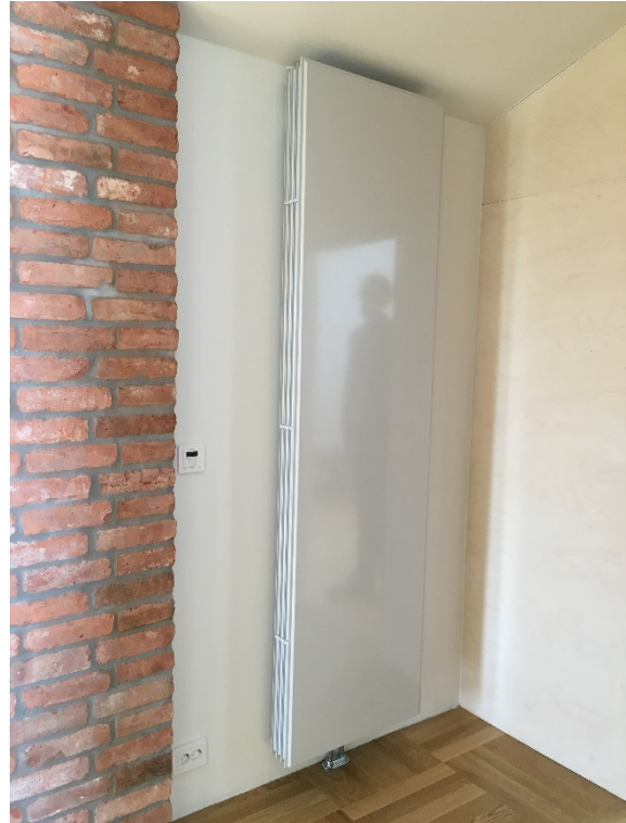
Figure 4.10 Radiator on the first floor (photo SINTEF)
