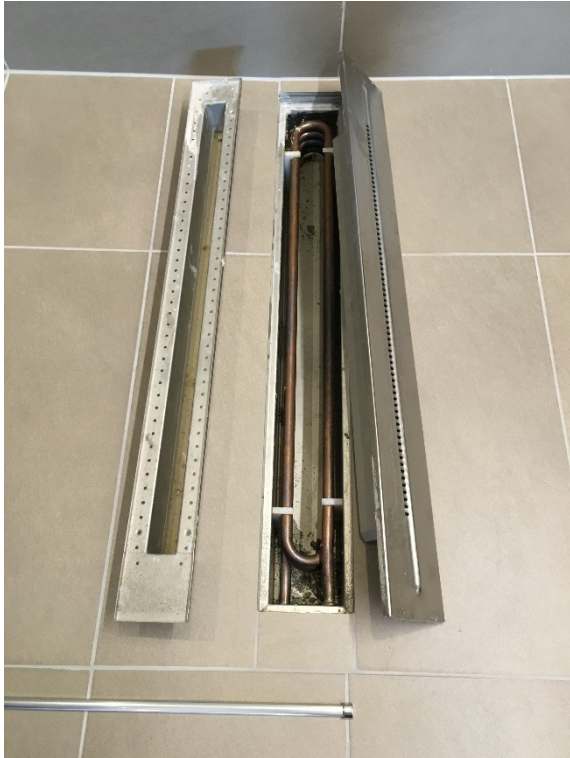
Figure 4.12 Grey water heat recovery system in the drain of the shower (photo SINTEF)
