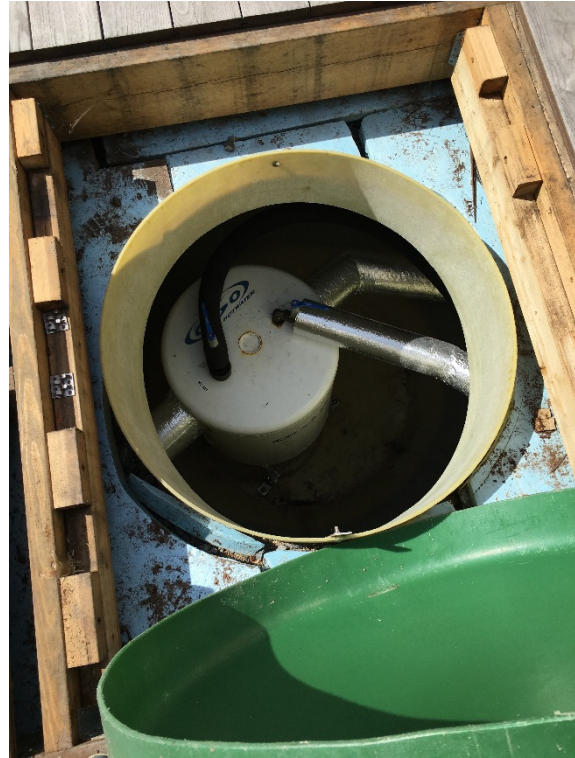
Figure 4.13 Grey water heat recovery system outside, including an accumulator tank (photo SINTEF)
