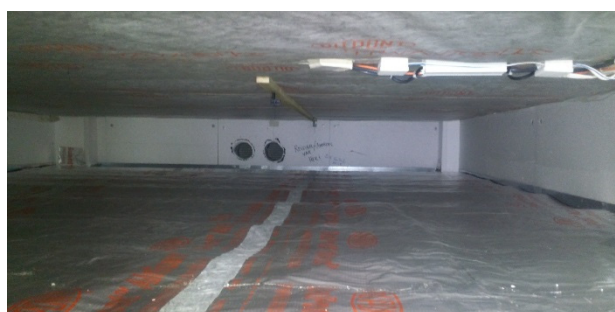
Figure 2.10 Crawl space with reflective foils and sensors mounted under the floor. Photo: SINTEF
