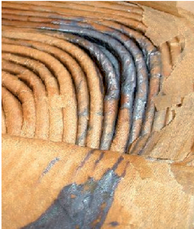
Figure 9. Picture of a part of a copper winding with paper from the transformer breakdown described in Chapter 1. From (Ohnstad 2005).
