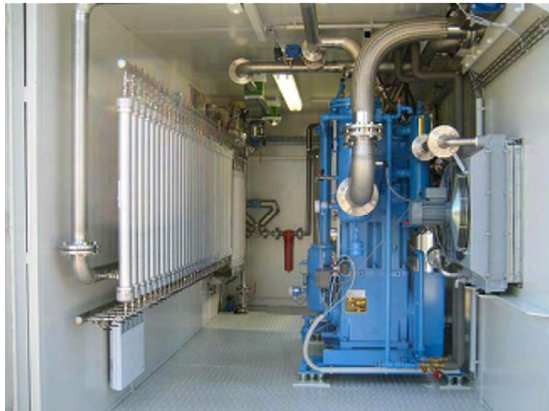
Figure 3.4 Interior of a membrane upgrading plant [7]
