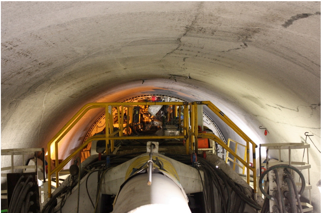
Figure 3: Boring of a headrace tunnel at the Røssåga hydropower project in 2013 represented the return of TBMs in Norway. The picture is taken towards the front of the Ø7.2 m TBM-O. Photo: Øyvind Dammyr
