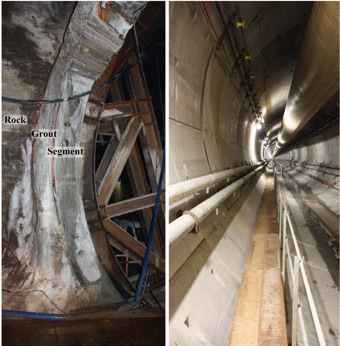
Figure 4: Observation of the rock-grout-segment interface of a single-shell segmental lining waterproofing concept (left). The picture was taken in a cross passage between the western and eastern tube of the Hallandsås tunnel in 2011. The segment thickness is 540 mm. The finished waterproof lining in the western tunnel is also shown (right). Photos: Øyvind Dammyr
