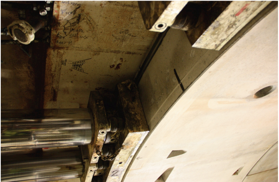
Figure 6: View of the L1* (forward working area) on the TBM-O at the Nant de Drance hydropower project in Switzerland (top) and the ring building area within the shield of the TBM-S at the Hallandsåsen tunnel project (bottom). Photos: Øyvind Dammyr
