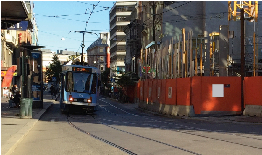
Fig. 1: Settlements induced by construction activity causes problems for the tramline in the street of Storgata (October 2015). Photo: Ø. Dammyr
