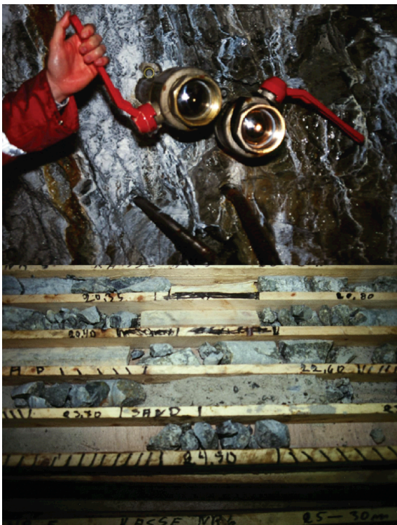
Fig. 5: View of part of the Bjorøy tunnel face after PEG with epoxy (top), and cores from core drilling at the face (bottom). Photos: B. Nilsen
