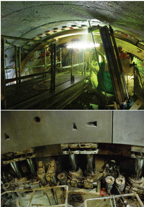
Fig. 6: The view at the rear of the shield at a TBM-O (top) and TBM-Slurry (bottom). Nant de Drance (Switzerland) and Hallandsås (Sweden) tunnel projects. The tunnels are ca. 9 m and 10 m in outer diameter respectively. Photos: Ø. Dammyr
