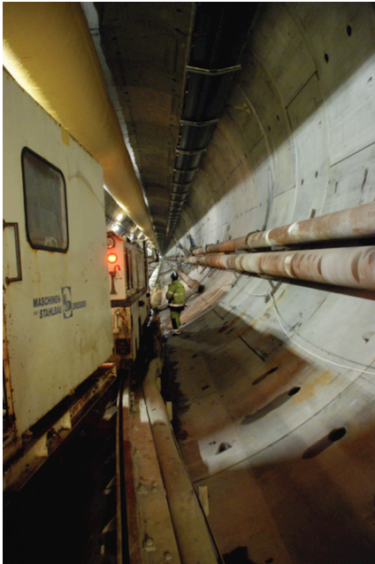
Fig. 6: Slurry transportation pipes, waterproof single shell segment lining and normal belt conveyor (for open mode tunneling) in the western-tube of the Hallandsås tunnel (Sweden). The inner diameter of the tunnel is 9 m. Photo: Ø. Dammyr
